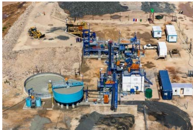
Bulk Sample Plant
